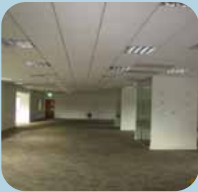
Original office space with inefficient lighting.
